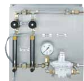
Gas supply system
