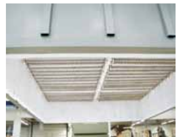
Heating elements in furnace hood
